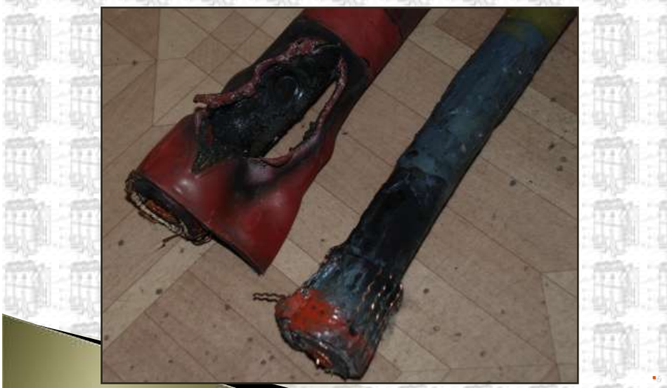
Damage of cable terminal at 35 kV VCB switching (Koksovaya Substation, Nizhny Tagil Steel Plant)
