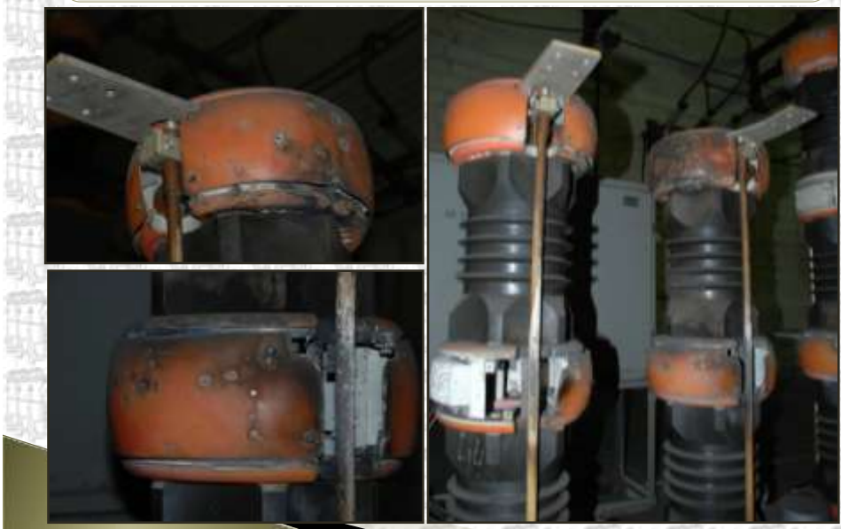
Damage of 35 kV VCB (Koksovaya Substation, Nizhny Tagil Steel Plant)
